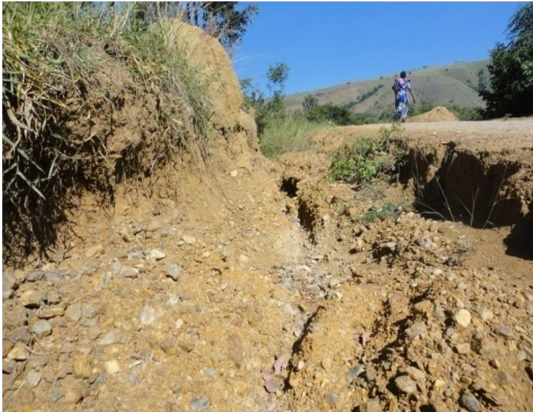
Plate 3. Heavily degraded section of one of the feeder roads, earth materials eroded are deposited in the wetland.
